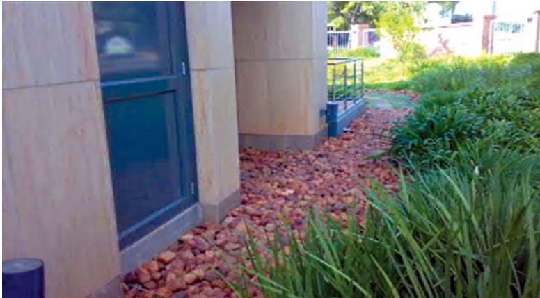
Figure 2. An exit door opens into a garden area layered with plants, rock and pebbles, and there's no safe escape walkway
